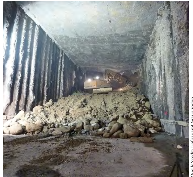
Querung in der Lockergesteinszone des Schanielatobel in Deckelbauweise Crossing the Schanielatobel soft ground zone was accomplished by cut and cover construction, using the top-down method
