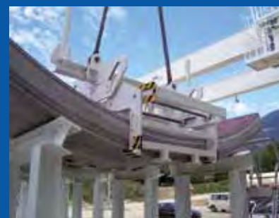
Segment handling system
