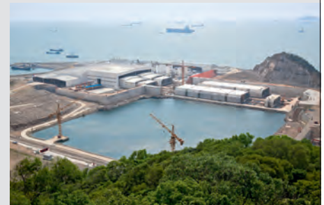
The 180 m long tunnel tube sections are pushed from the field factory into a dry dock, sealed by means of bulkheads, flooded and then towed to their final positions.
