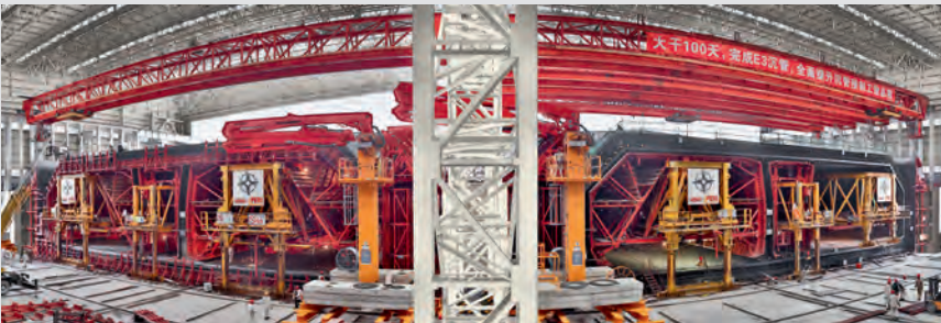
Two hydraulically-operated shuttering machines are being used for the efficient realization of 33 tunnel elements with a length of 180 m using the incremental launching method.
