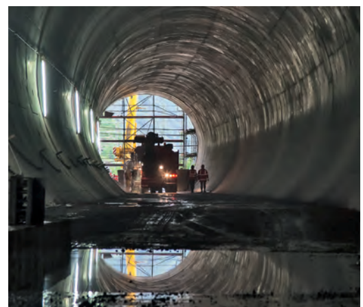
Tunnelansicht NKWT innen Blick Richtung Cochem View inside the NKWT towards Cochem
