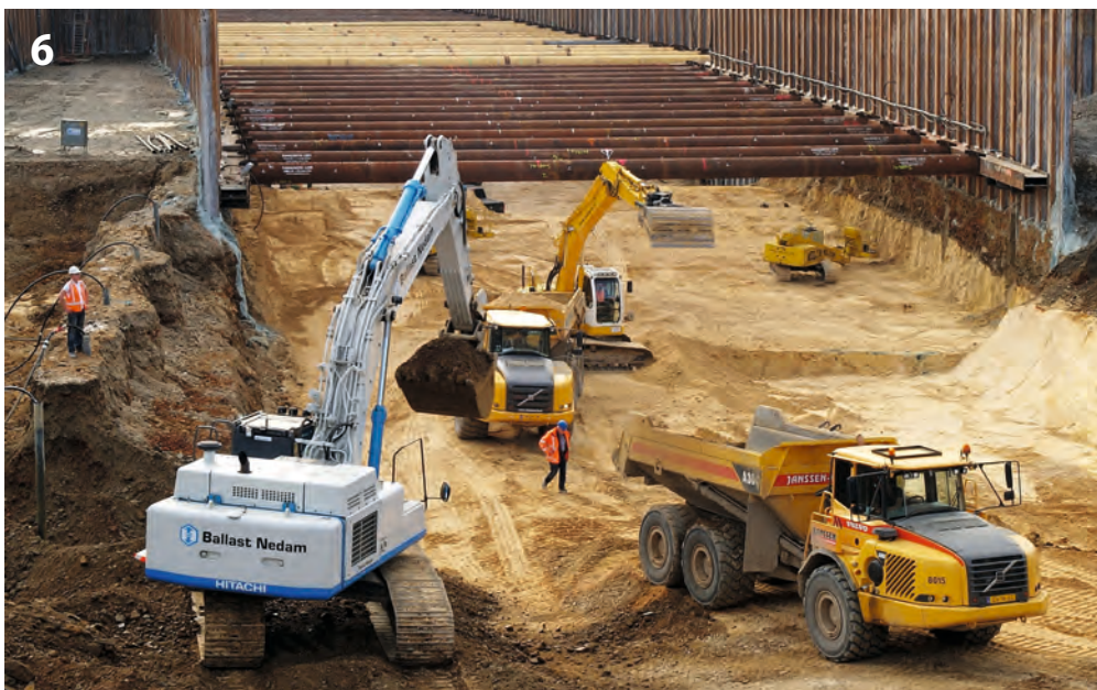
Blick in die Baugrube während der Erdarbeiten View of the excavation pit during the earthworks
