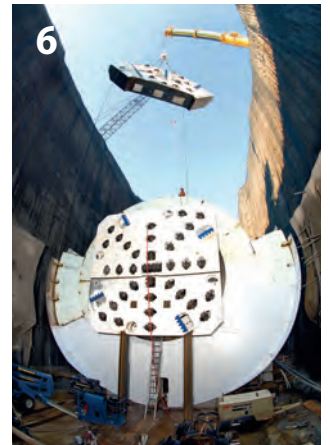
Robbins developed its successful Onsite First Time Assembly (OFTA) method for the Niagara Tunnel Project in 2006
