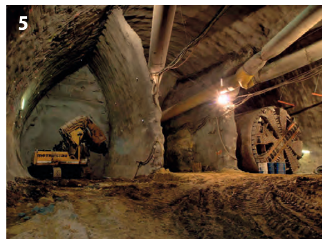
The side-drifts of Petriny Station were filled with light concrete to form a vertical wall for the EPBM breakthrough
