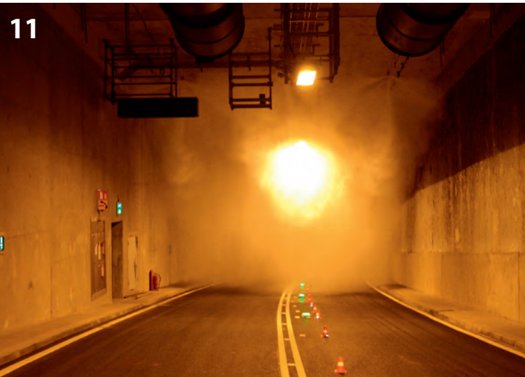
Commissioning the test of FFFS in the new Tyne Tunnel in February 2011 [8]
